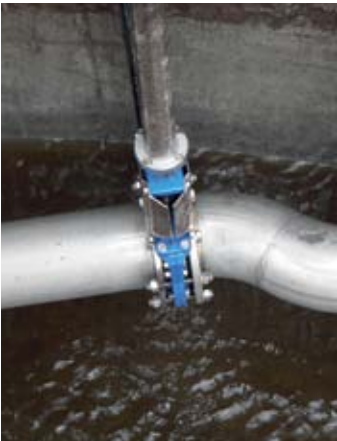
Wastewater treatment plant Seebergen, Germany VAG ZETA® Knife Gate Valves
