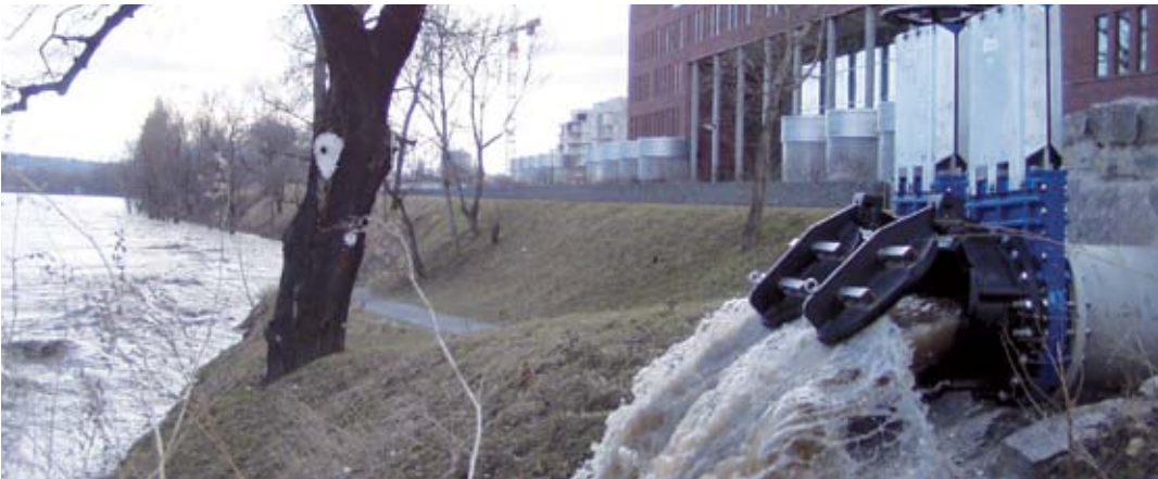
Flood protection of Prague, Czech Republic VAG HADE® Non-Return Valves with VAG ZETA® Knife Gate Valves
